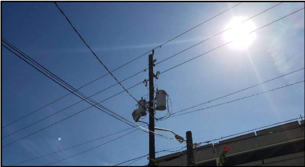
Pole-mounted transformers located at the South-East corner of the subject property. No evidence of corrosion or leakage was found.
